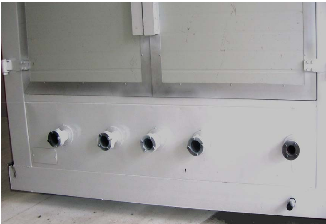
(4) Fuel, Oil and Water (without radiator) Pipe system
